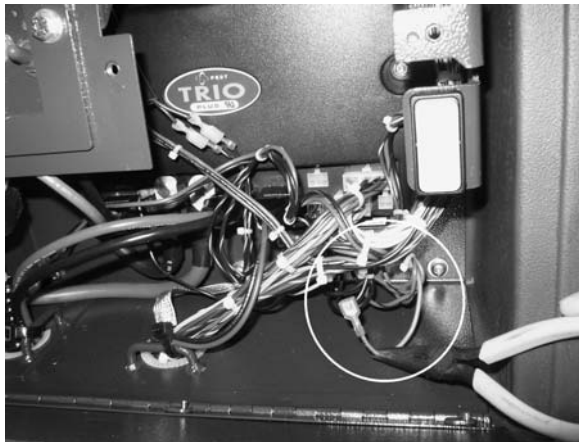
Figure 1 Jumper wire disconnected
